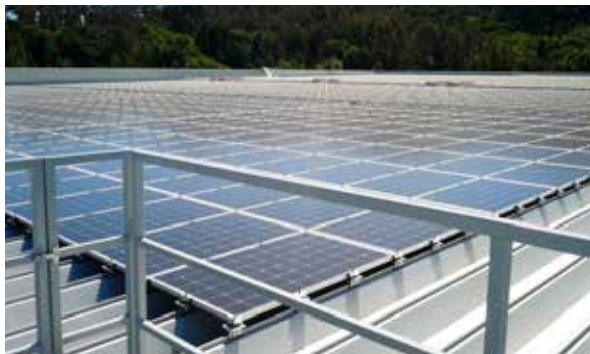
Solar panels at Fujiyama Works
