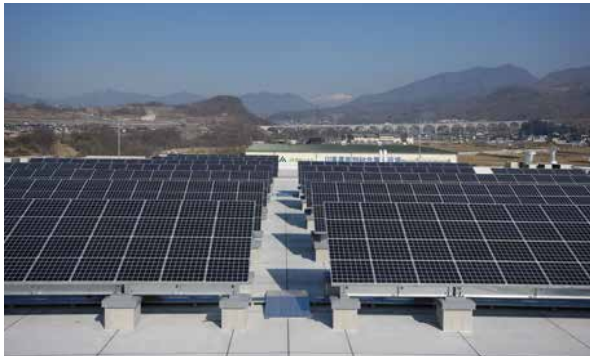
Solar panels at Kangawa Works
