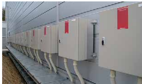
PV Inverters at Fujiyama Works
