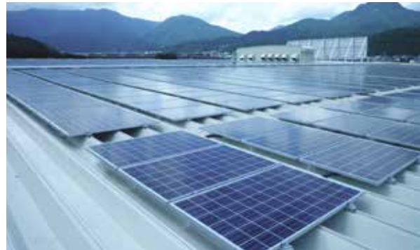
Solar panels at Logistics Center
